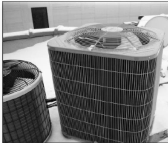
Air conditioning systems
